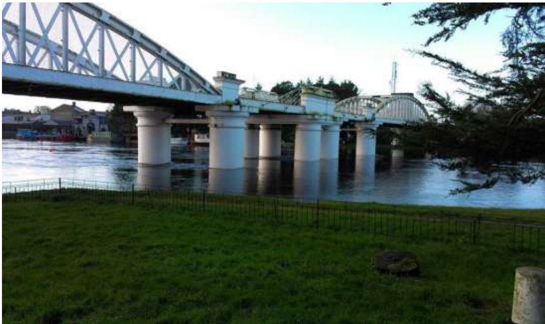
Plate 3.3 View of the north side of the Railway Bridge from Marine View, east bank
